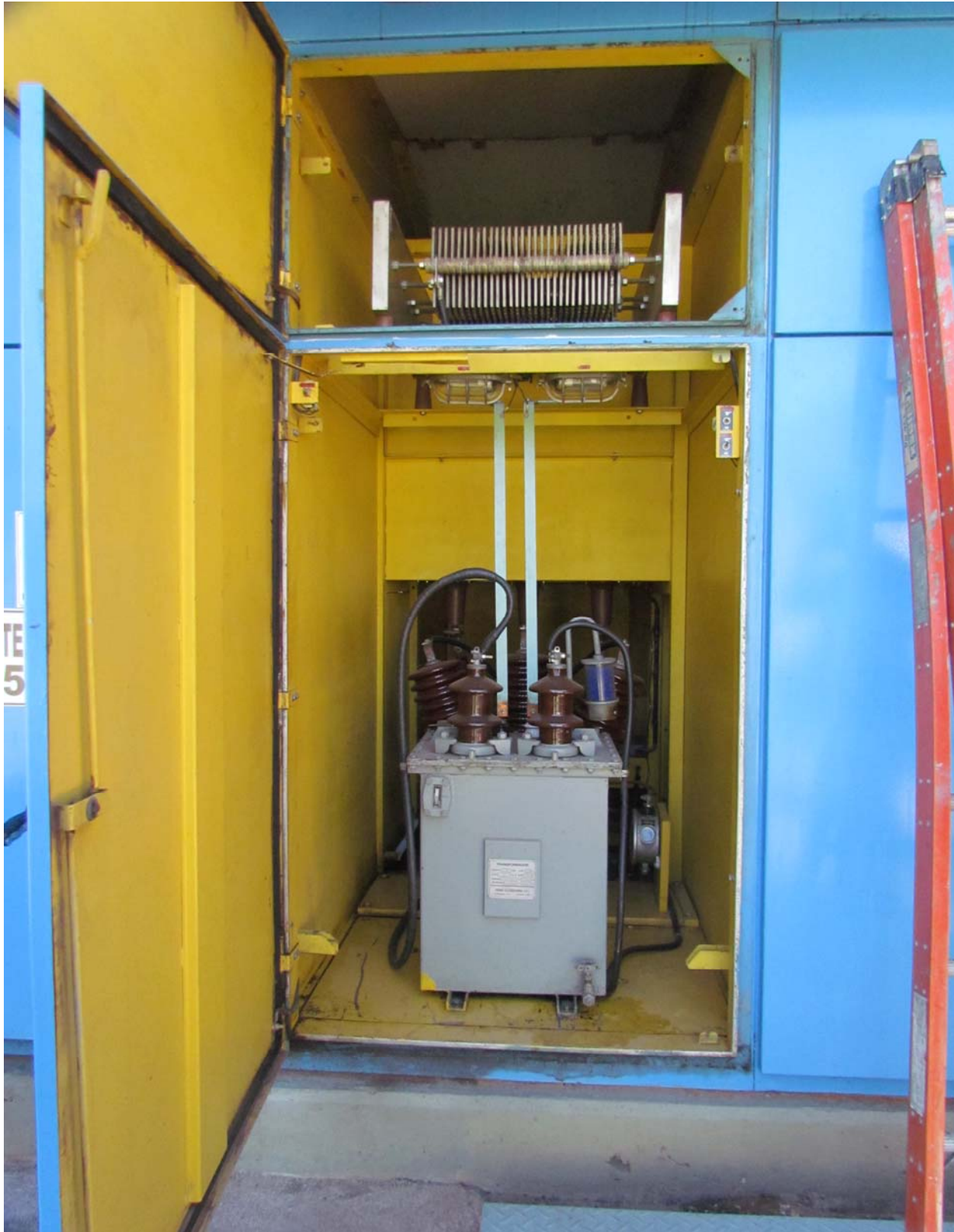
Neutral Grounding Transformer and Neutral Ground Resistor
